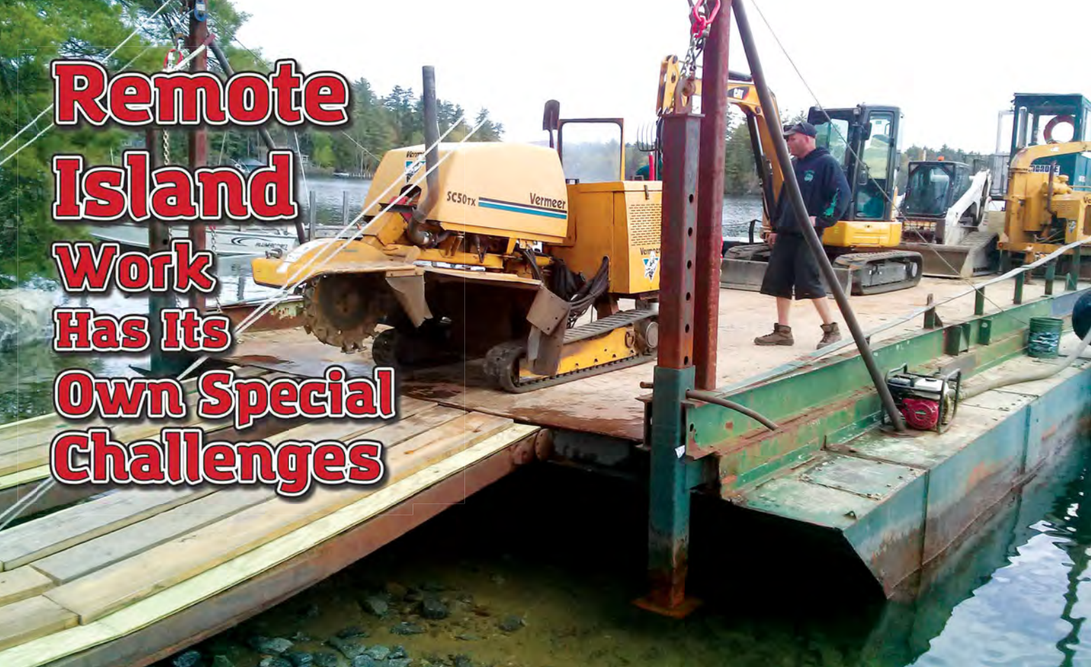
A crew member from Belknap Landscape Company unloading a stump grinder from a barge at a property on Lake Winnepesaukee in Meredith, New Hampshire. Courtesy of Belknap Landscape.
